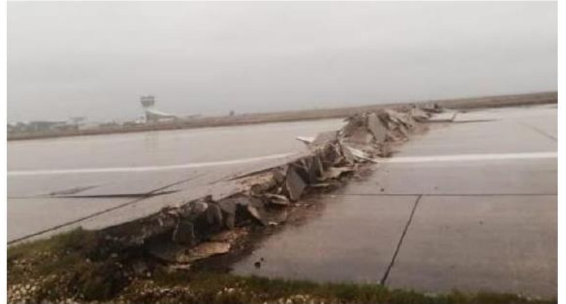
Runway buckled at Hatay Airport
