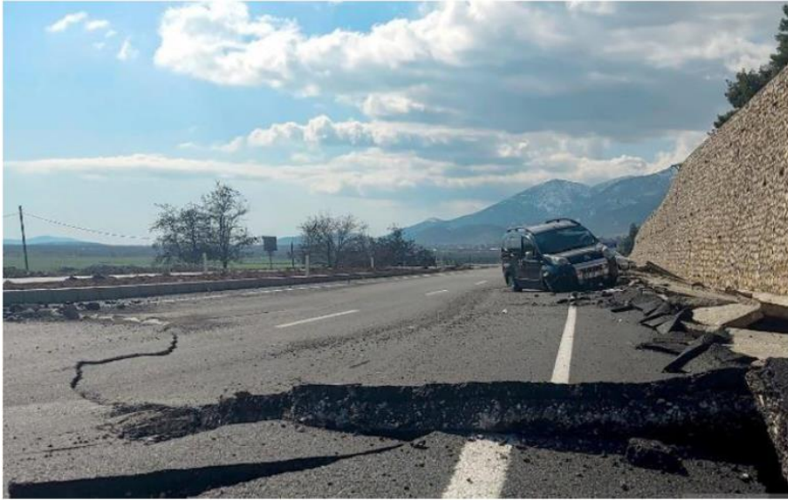
Roadway pavement failure
