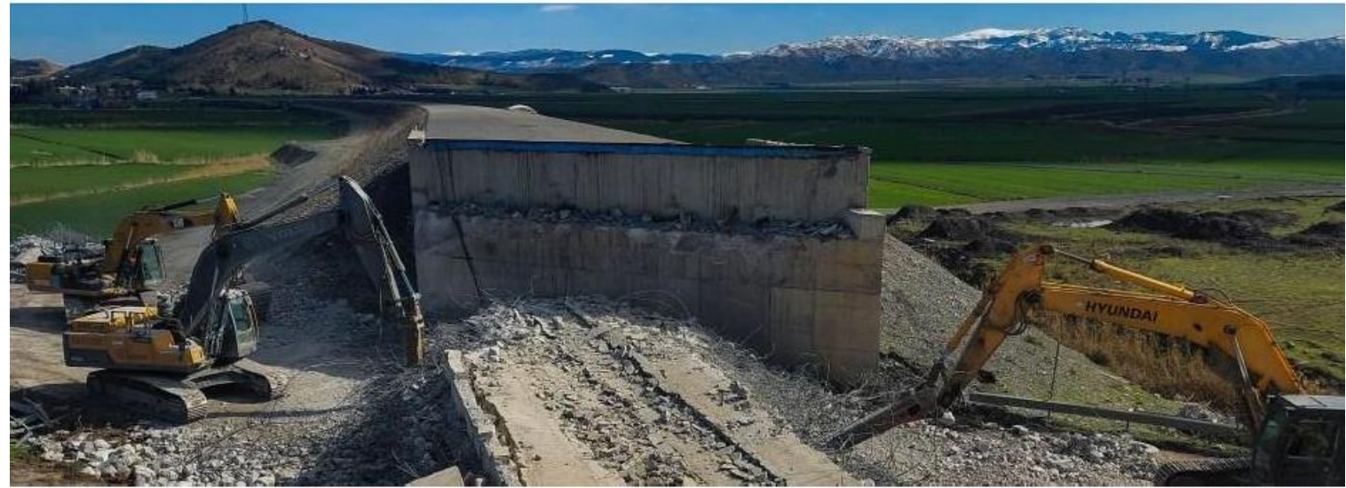
Bridge superstructure failure
