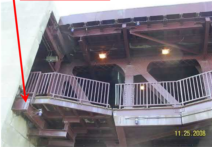
1980s hinged sidewalk, closed position
